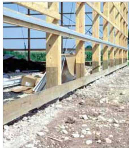
Figure 12. Laminated columns often splice treated wood on the bottom end to untreated wood above grade.
